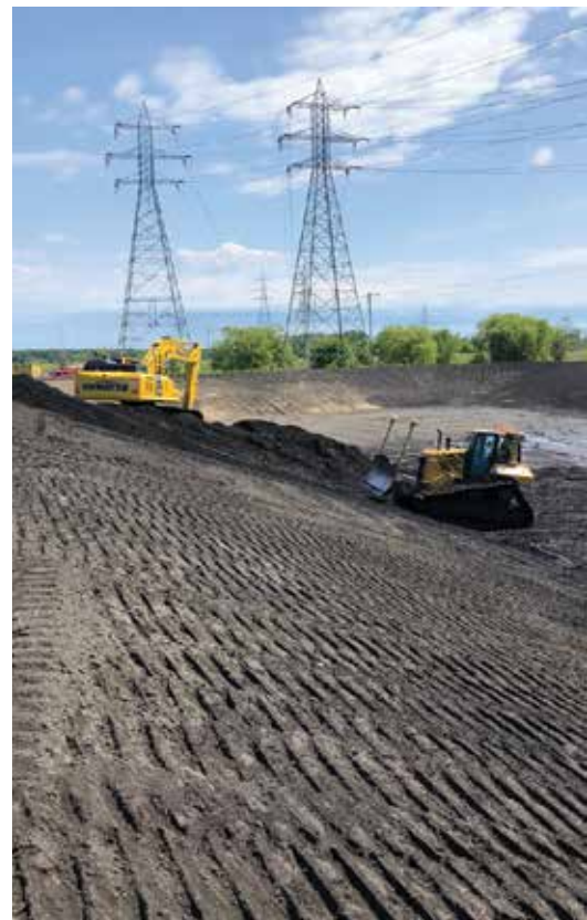
Ash being excavated from B.C. Cobb ash ponds in preparation for pond closure.
